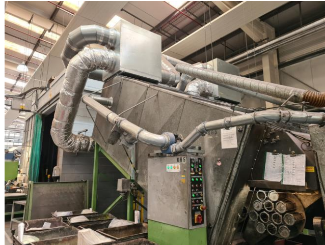
Heat exchanger fitted to the strip oven (left)
